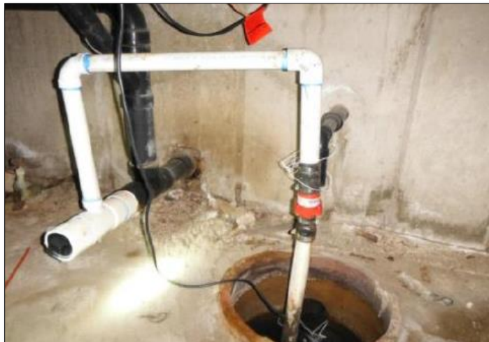
Figure 17: Illegal Sump Pump Connection to a Sewer Service
