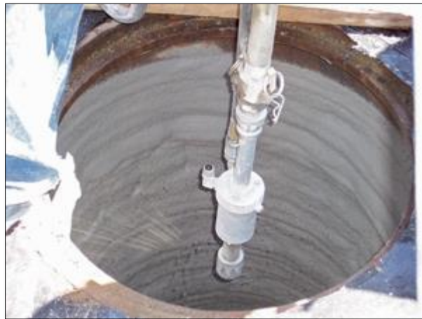
Figure 19: Monolithic Cementitious Manhole Liner
